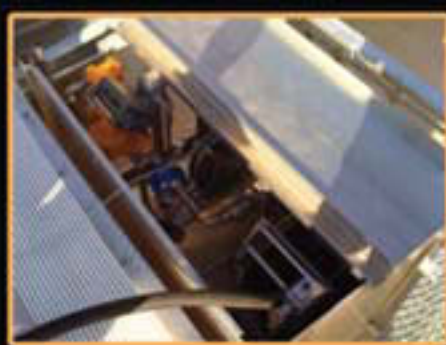
St. Mary's Hospital, Grand Junction, CO Rooftop Helifuel Dispenser
